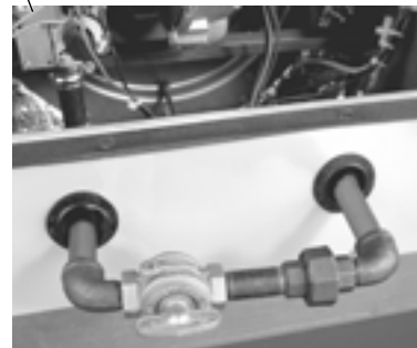
Through the Base Gas Piping
